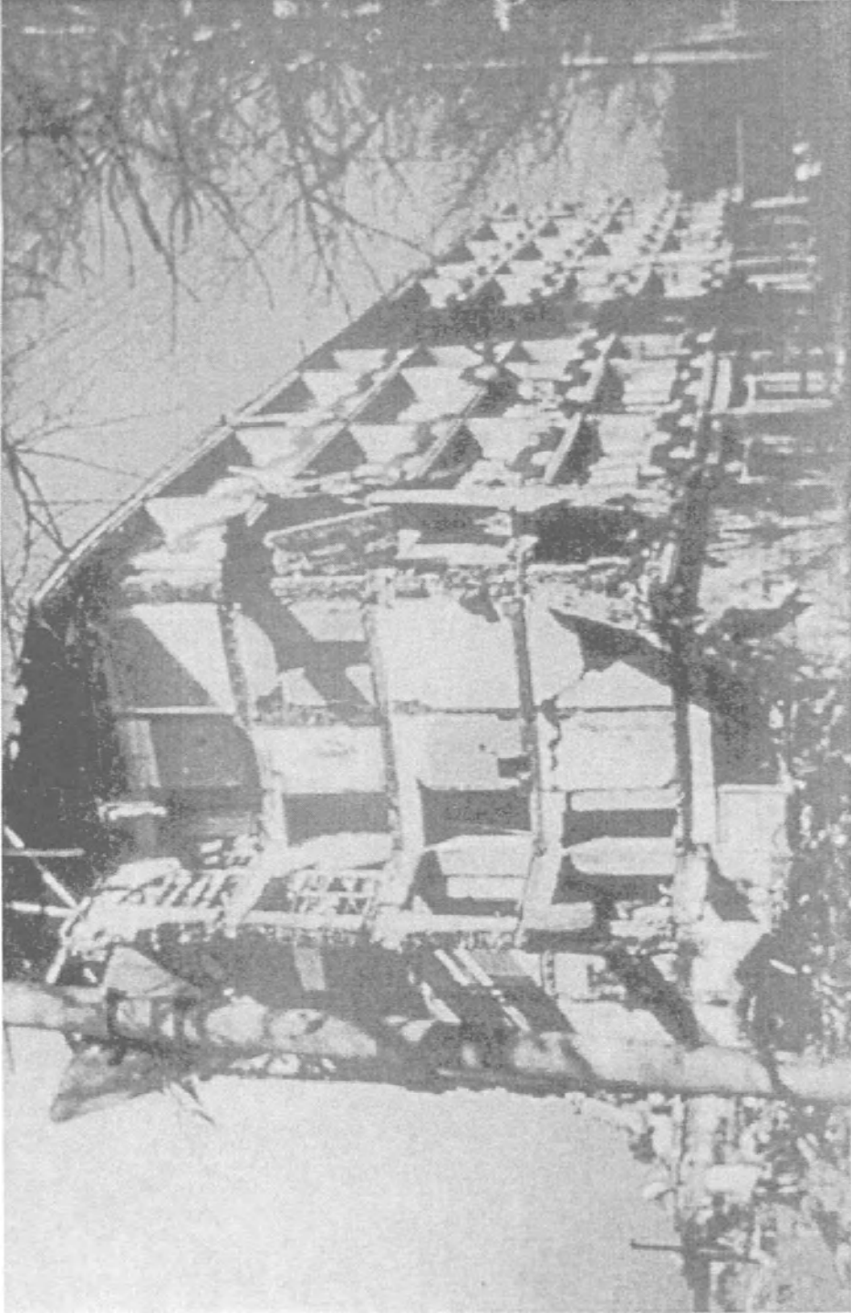
Figure 6. Damage to side section of residential house of series 1A-450.
